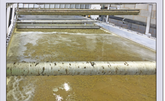
A reliable solution to a previously problematic sludge and scum transfer system.
